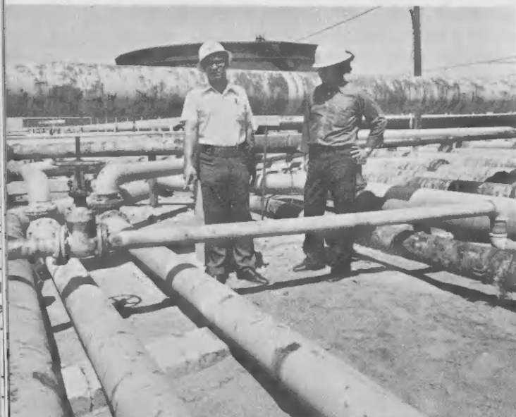
Vicente Thiel shows here where ■ leak problem was eliminated by installation of a new pipe ■■ the Gasoline Pumphouse..
